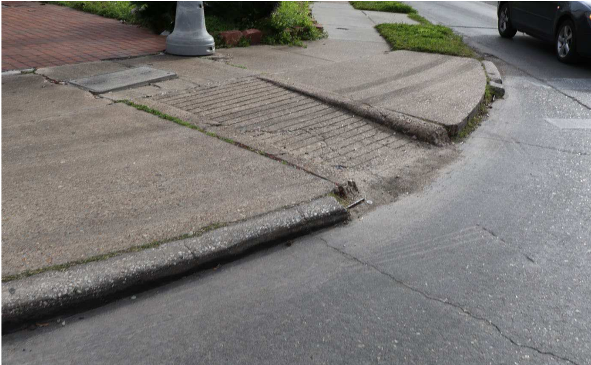
Figure 17: Broken curb, vehicle off-tracking, and sidewalk condition.
